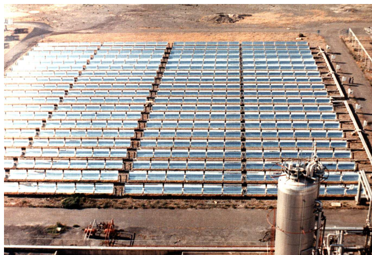
Figure 1.3: View of the ACUREX solar field.
