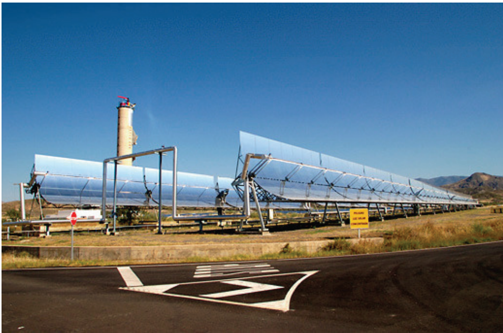
Figure 3.11: General view of the DISS test facility
